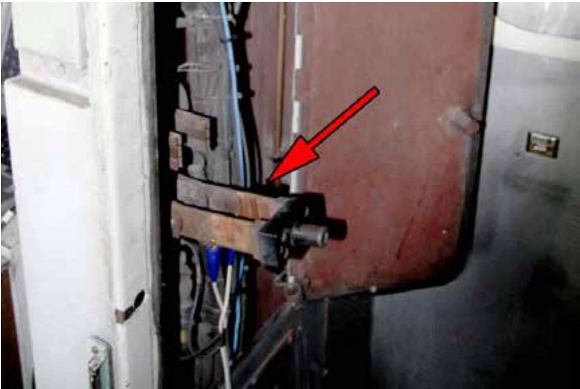
Figure 5: Main electrical cut-off switch
