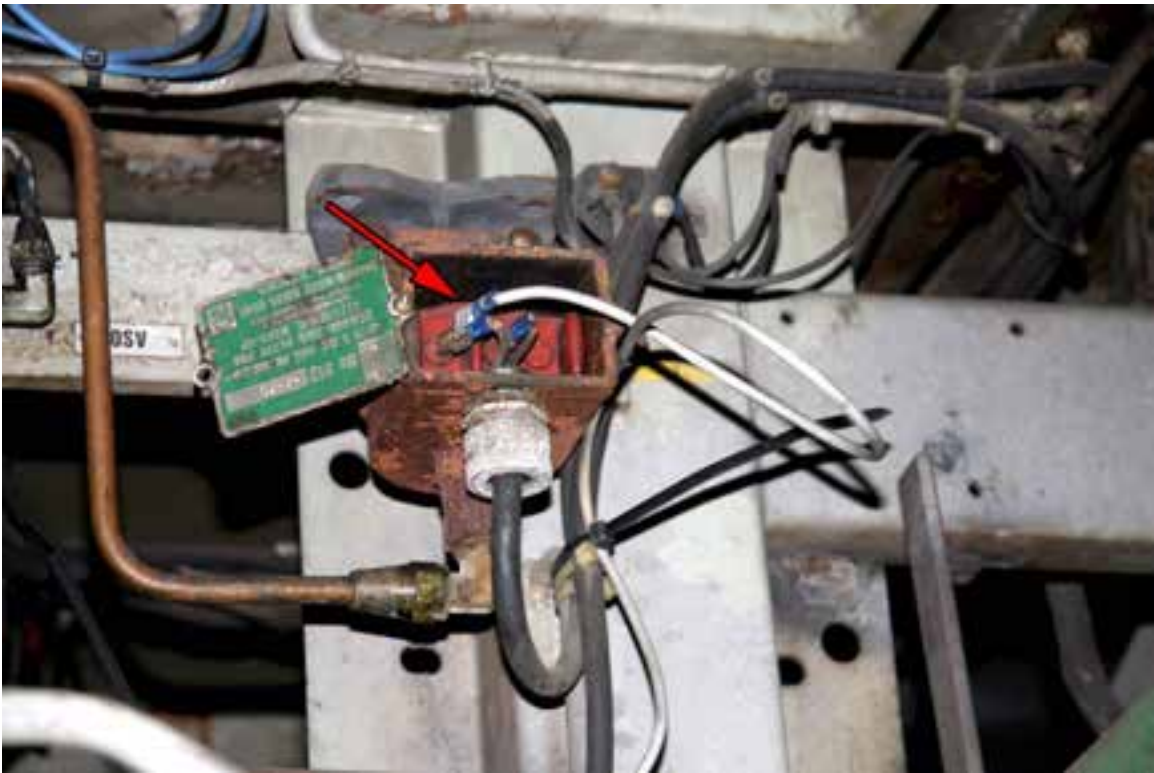
Figure 3: "Brake Test" connection for locomotive 5017
