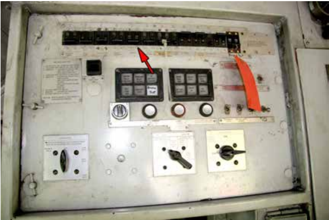
Figure 4: Control circuit breaker in locomotive cab
