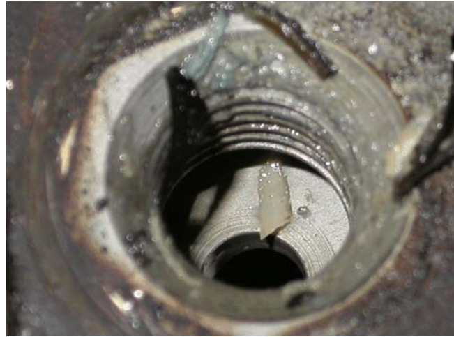
Photo 1. Piece of thread sealant in valve seat
