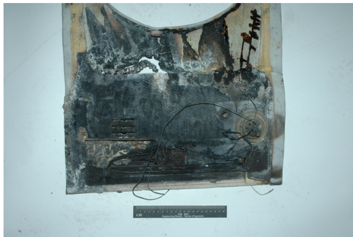
Photo 4. Interior of panel LH/4 indicating where the power supply melted and burned
