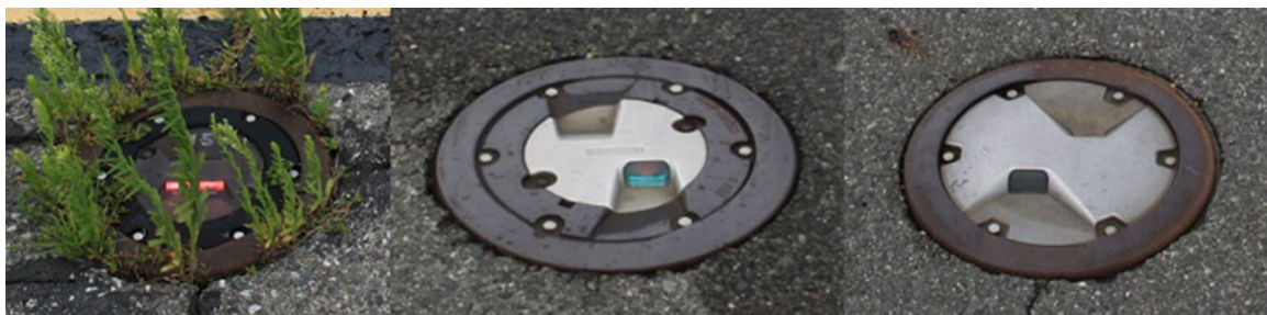
Figure 16. Composite image showing obscured lights, incorrect lenses, and non-functioning bulbs at Runway 06L/24R
