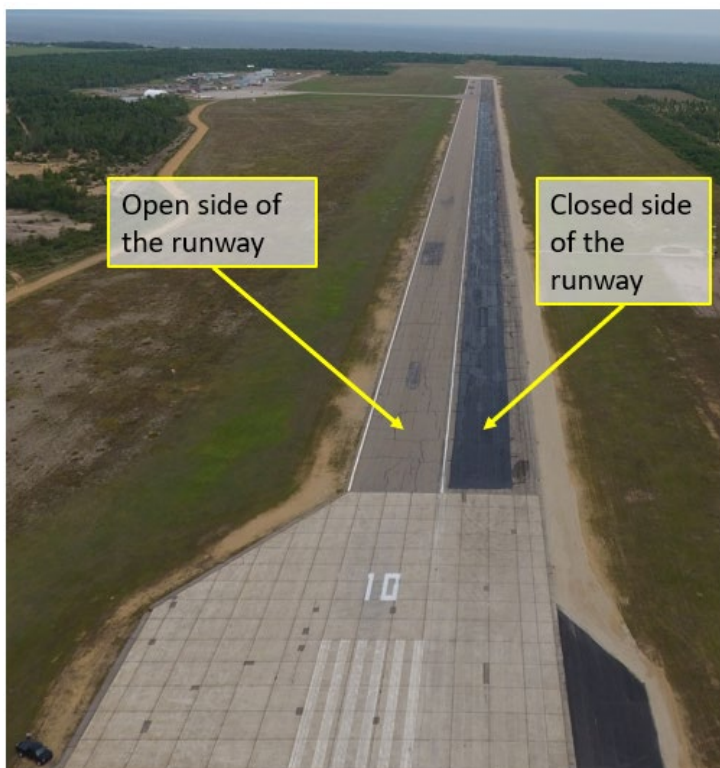
Figure 5. Aerial photo of Runway 10 at the Baie-Comeau Airport during the rehabilitation work on the south side of the runway in June 2018 (Source: Baie-Comeau Airport, with TSB annotations)
