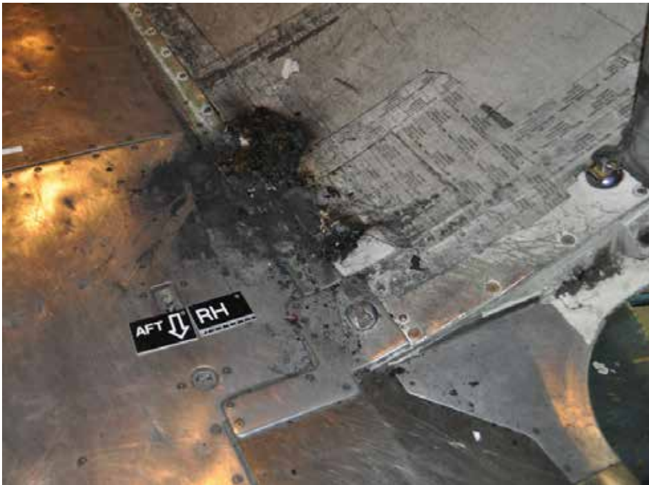
Figure 2. Fire damage to lower aft cargo compartment
