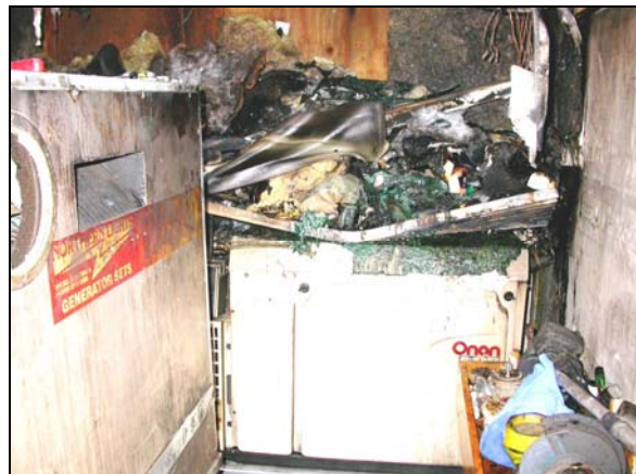
Photo 3. Collapsed shelf in engine room where flammable goods were stored
