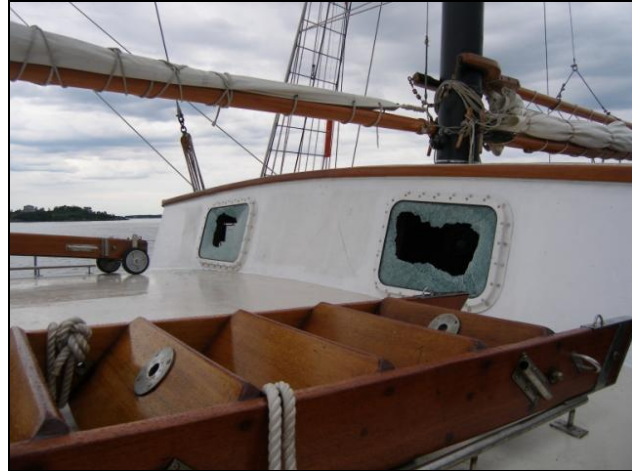
Photo 2. Front windows of the deckhouse broken by firefighters (to ventilate the accommodation area)
