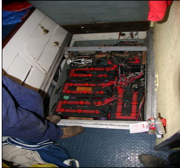
Photo 8. Floor compartment housing the main house-and-electronic battery bank
