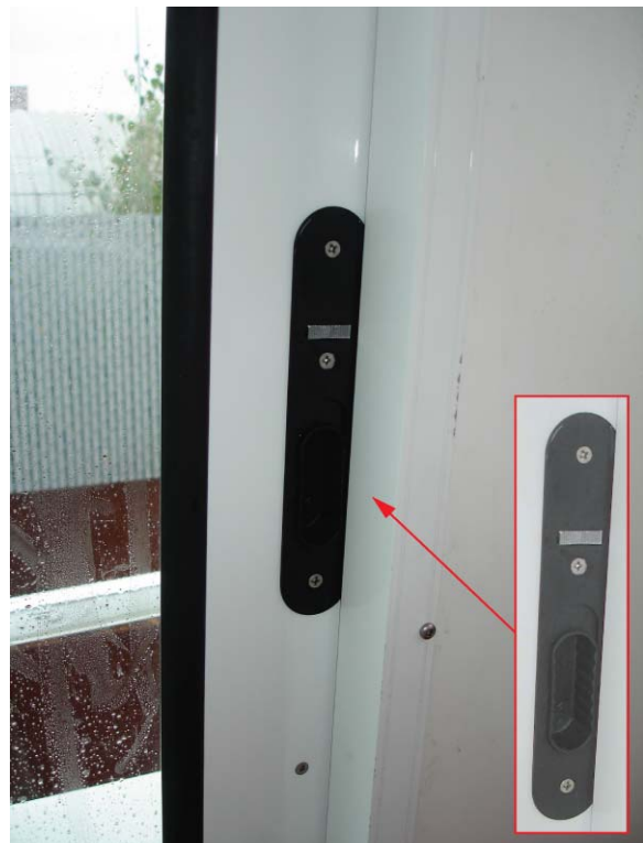
Photo 5. Starboard door interior latch (note position difference from port door latch)
