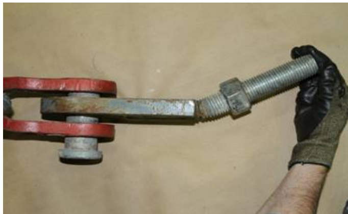
Photo 7. West cable, north anchor showing approximate deformation in the downriver direction before fracture
