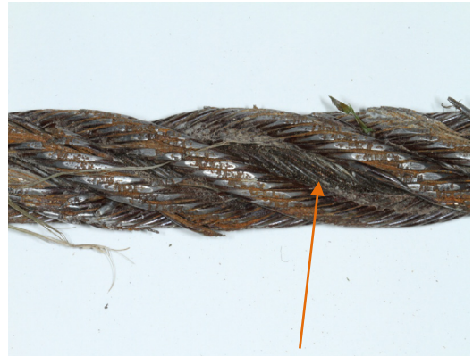
Photo 2. A section from the east cable showing the core strand exposed due to a missing strand
