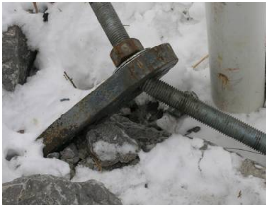
Photo 6. Close-up of deformation to the west cable, south anchor assembly; this shore attachment did not fail
