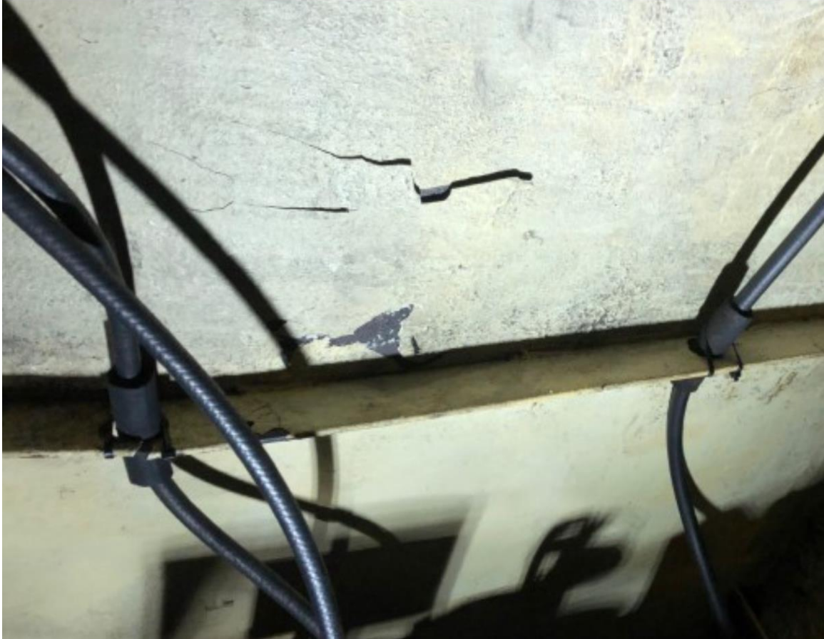
Figure 7. Damage to the structural frame and bulkhead that separated the battery compartment from the engine room (Source: Glory Days Towing Ltd.)
