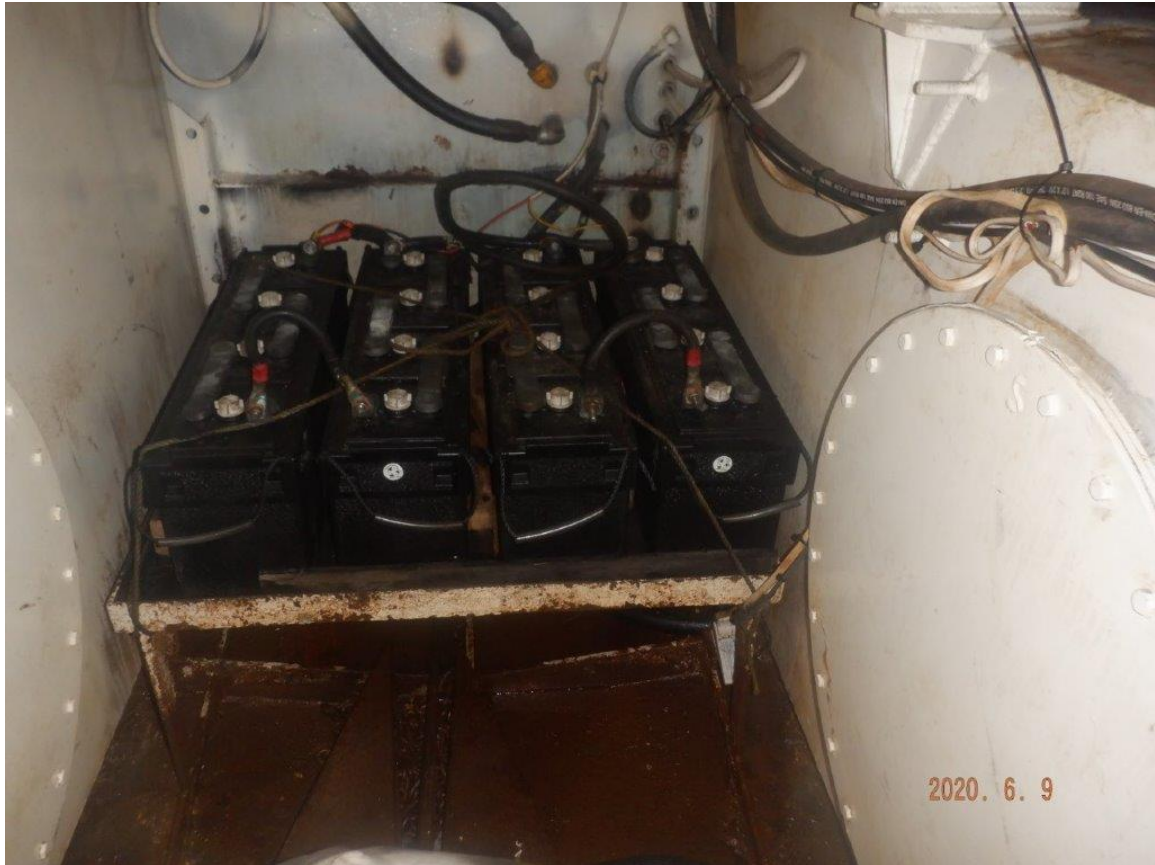
Figure 4. A photo taken 2 months before the occurrence shows the battery bank of four 8-VDC batteries located in the forward part of the lazarette in between 2 fuel tanks (Source: Accurate Appraisals & Marine Surveys Ltd.)
