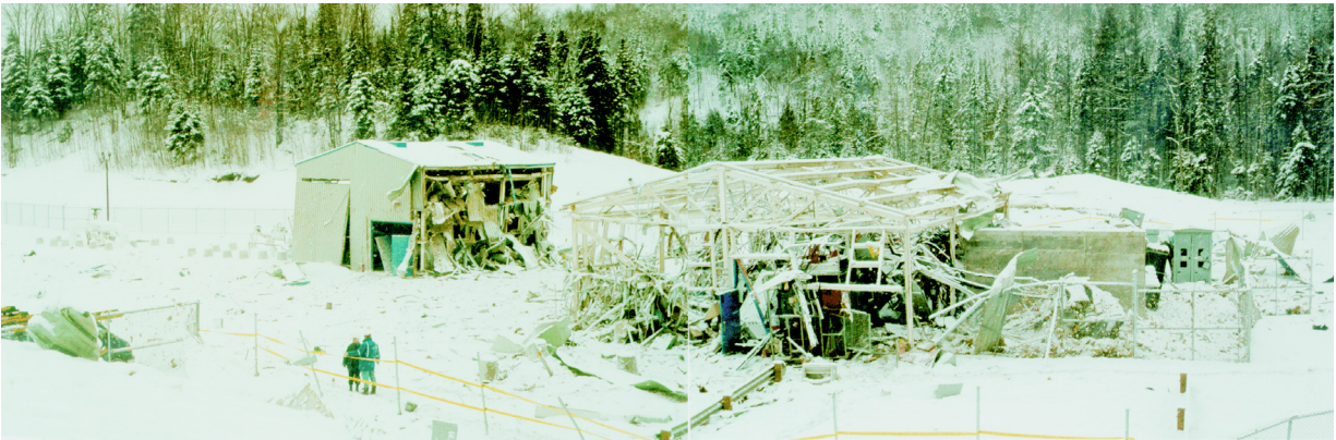
Photo 1. Panoramic view of East Hereford compressor station (after explosion)
