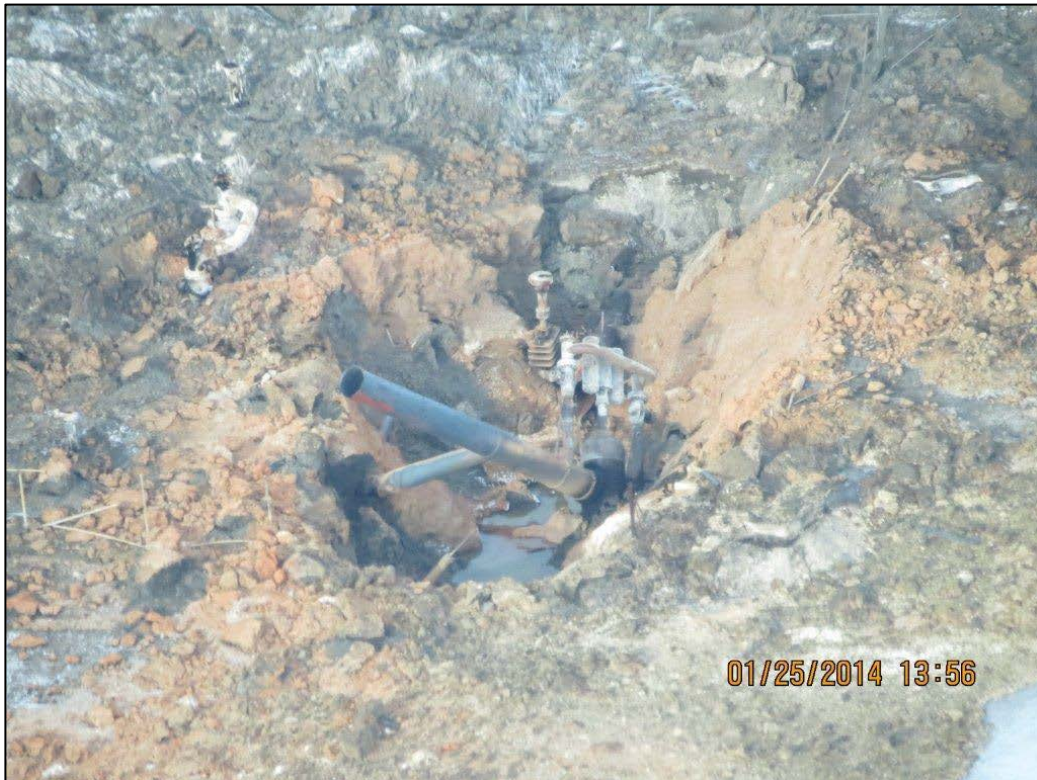
Photo 1. Pipeline failure damage
