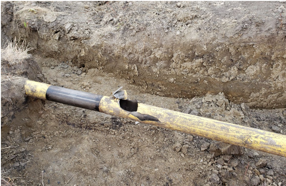
Figure 4. Excavated area showing the damaged section of pipeline (Source: TSB)
