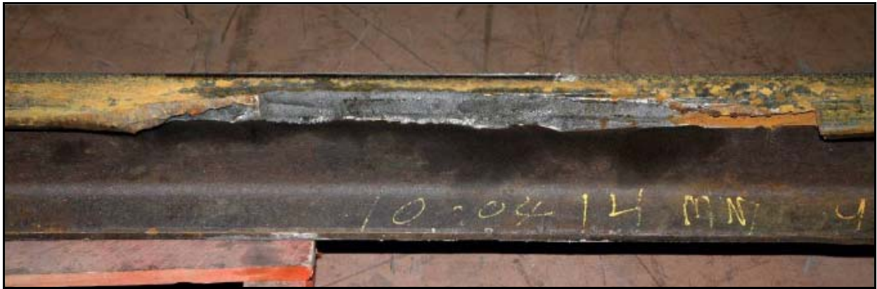
Photo 2. Vertical split in the rail head of the Dominion plug rail
