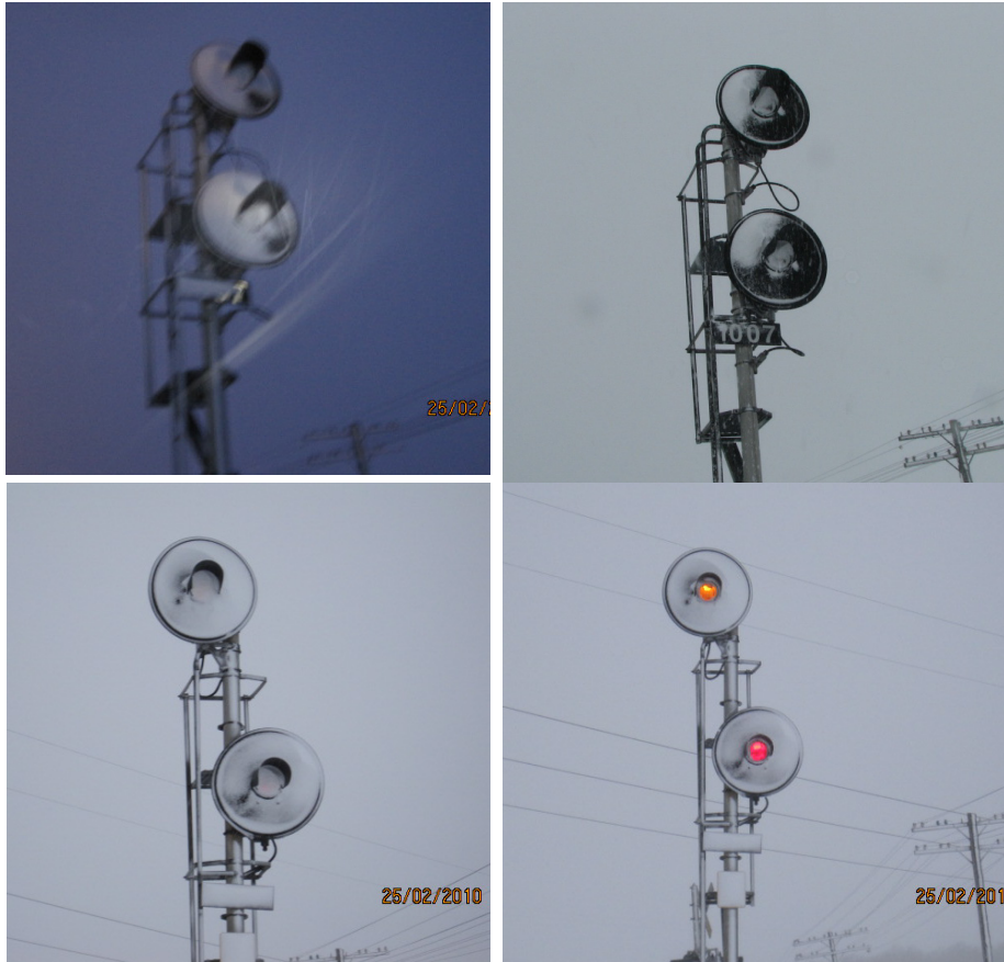
Photo 2. Top: Snow on signal lenses at home signal 1007 (25 February 2010 at 0700 and 1130). Bottom: Advance signal 971 before and after cleaning lenses (Source: TSB and CN)
