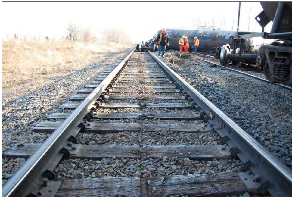
Photo 4. Looking north, wheel marks on main-track ties north of the switch
