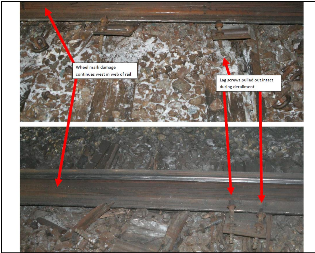
Photo 1. Track damage on high rail
