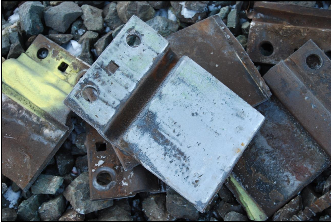
Photo 8. Shiny bottom of broken rolled plate
