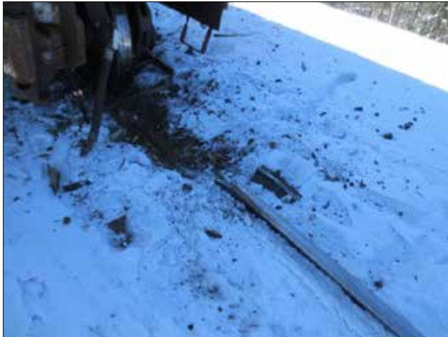
Photo 1. Broken south rail at Mile 9.41 (looking east)
