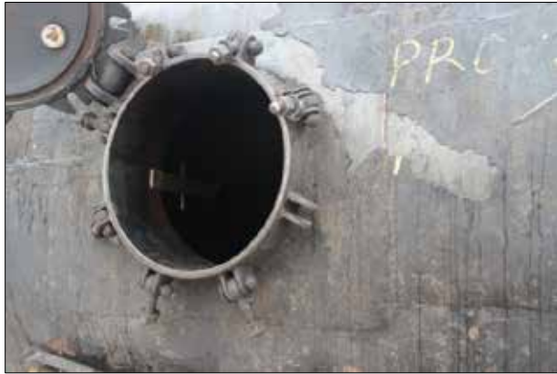
Photo 9. Missing manway tie-down
