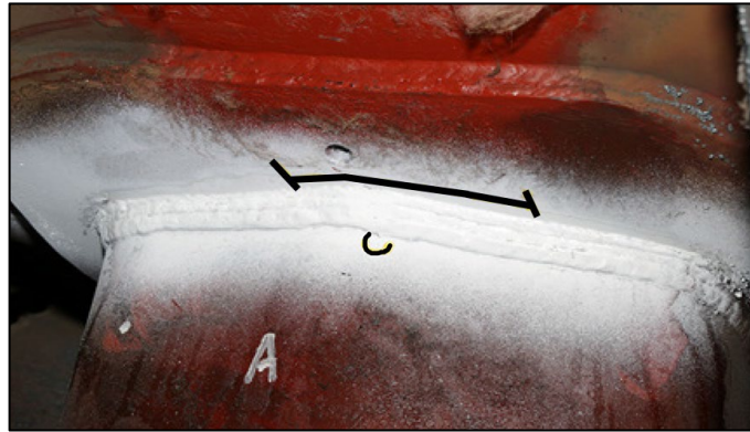
Figure 7. Location of cracking observed in A-end of car TGOX 155010 head brace weld outlined in black
