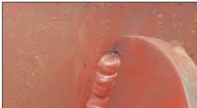
Figure 8. Close-up of crack in weld at body bolster extension / bolster pad junction
