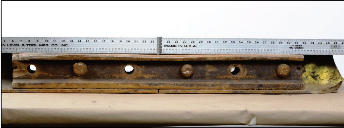
Figure 6. Gauge joint bar with missing bolts
