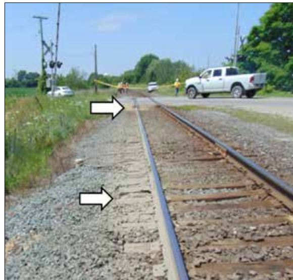
Figure 8. Mud contamination on the east side of the Carroll Street East crossing, looking west
