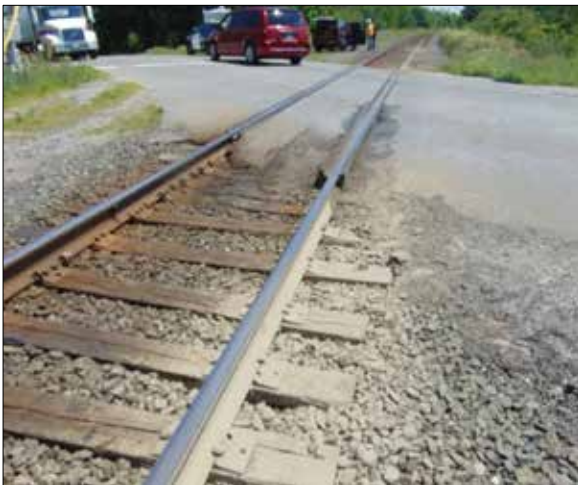
Figure 7. Mud contamination on the west side of the Carroll Street East crossing, looking east
