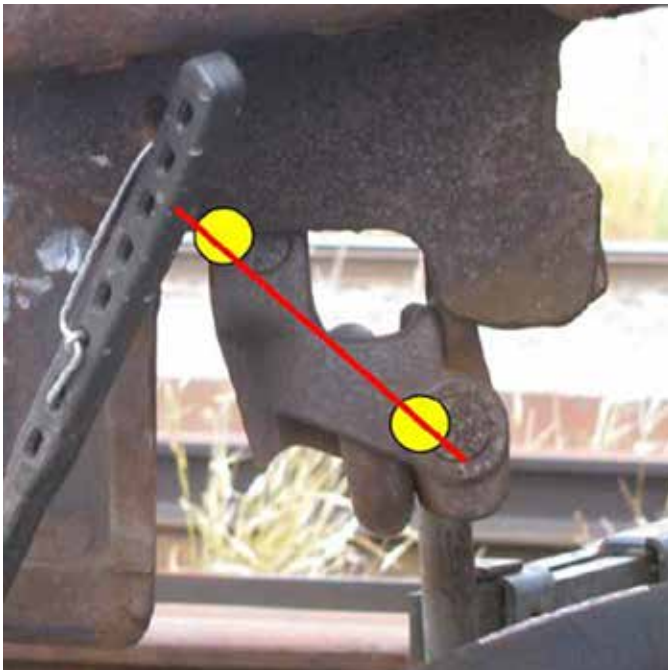
Figure 26. Misalignment of the lock-lift assembly pivot points in a bottom-operated lock (locking block not fully dropped) (Source: Canadian National Railway Company)
